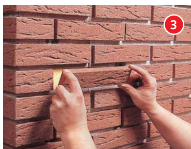
The recessed bricks are glued into the connection points for the individual elements to complete the connection.
